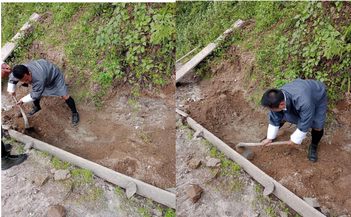
Site engineer showing an example as to how the foundation of the drain should be laid
