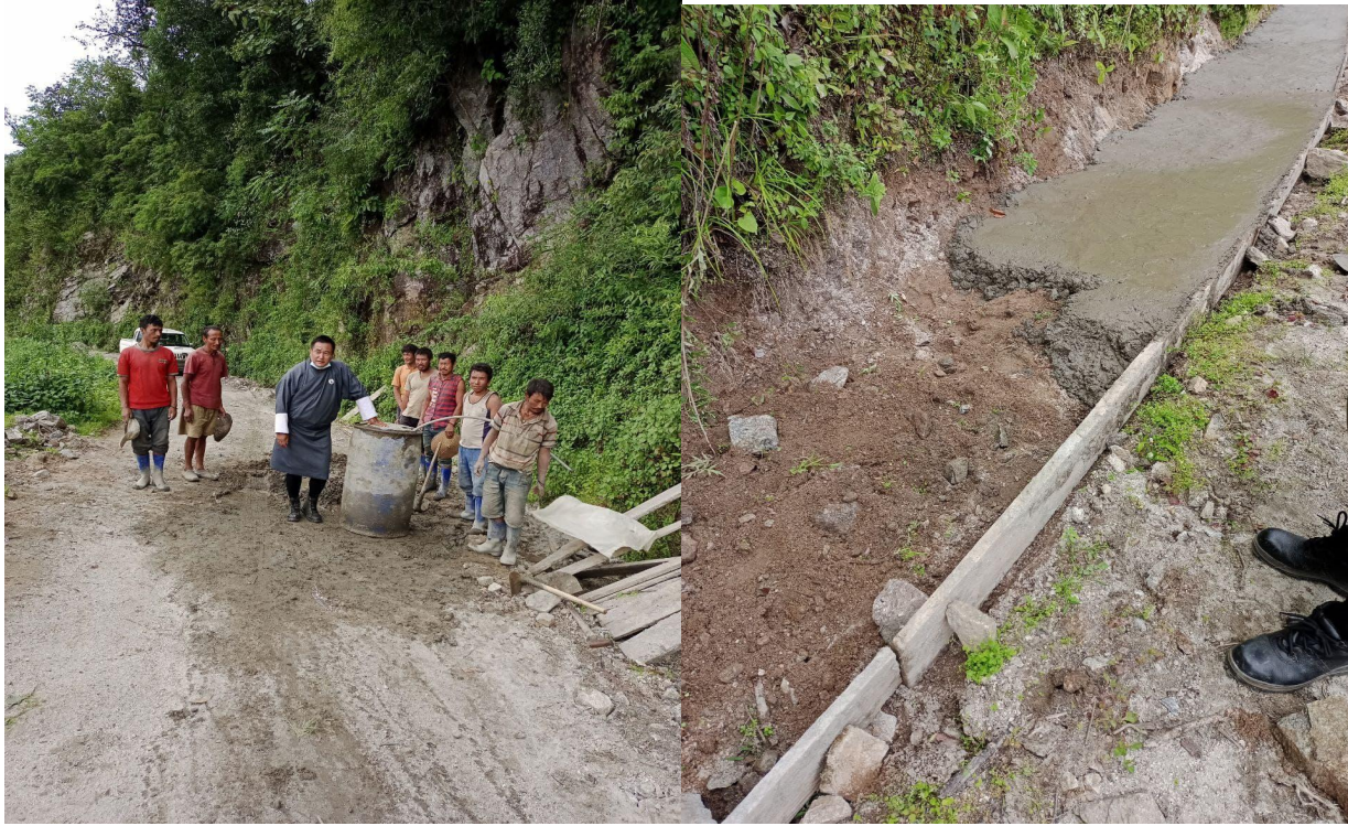
With Labourers at the ongoing construction of drains at Bardo GC road blacktopping
